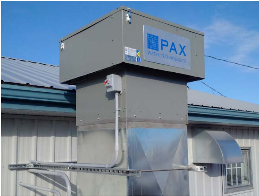
The team factored in the sub-zero temperatures during the Manitoba winter and added an air heater to the Powervent ventilation unit.
