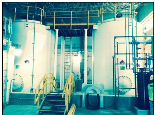
Hypochlorite (Bleach) Storage Tanks
